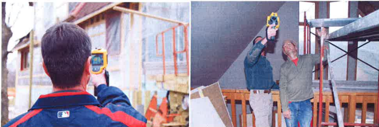
Thermal imaging was used to verify the thoroughness of construction both inside and out.
