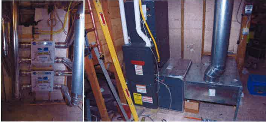
An air handling system is an important component of an air tight building.
