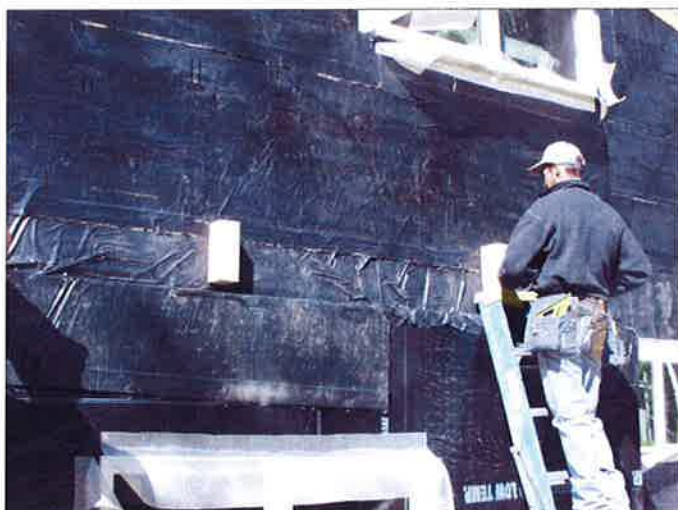
REMOTE wall under construction showing exterior vapor barrier, deck blocking & window detail.
