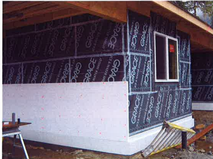
A house using the REMOTE wall system building technique under construction in Juneau, Alaska.
