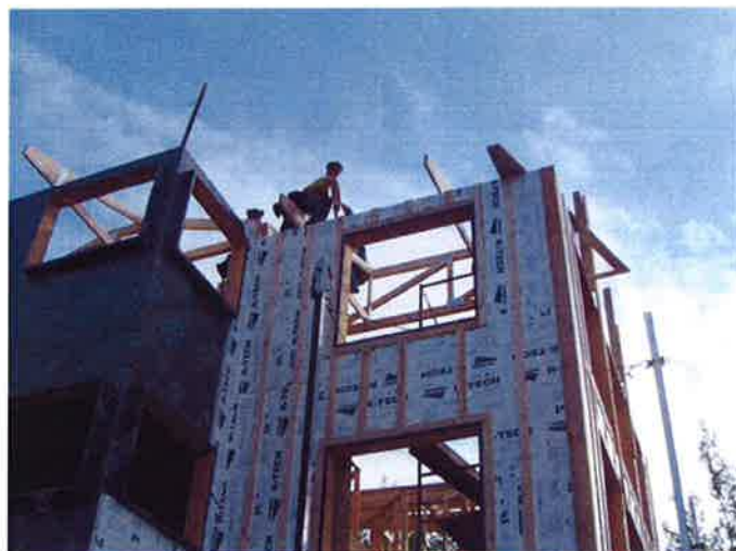
REMOTE wall under construction in Fairbanks, Alaska showing vapor barrier, insulation, window framing and furring in place for siding.
